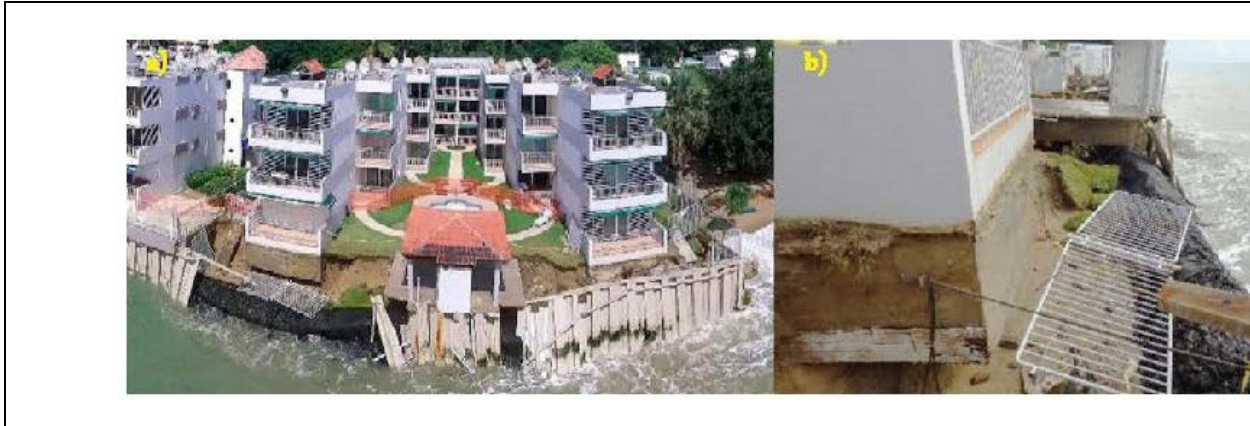
Figure 2-15. a) Damages to the Rincón Ocean Club 2 condominium caused by Hurricane Matthew, September 2016. b) Close view of failed seawall and exposed foundation
